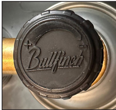
Gas Manifold Valve (Open and Close)
