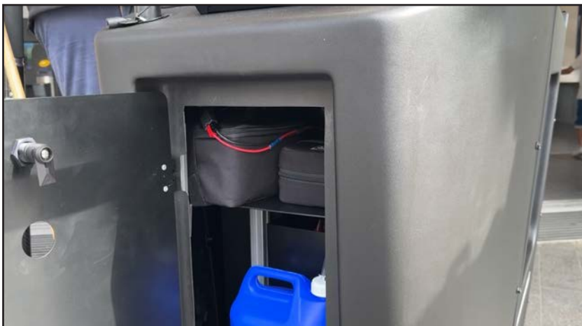
Both Batteries Installed
